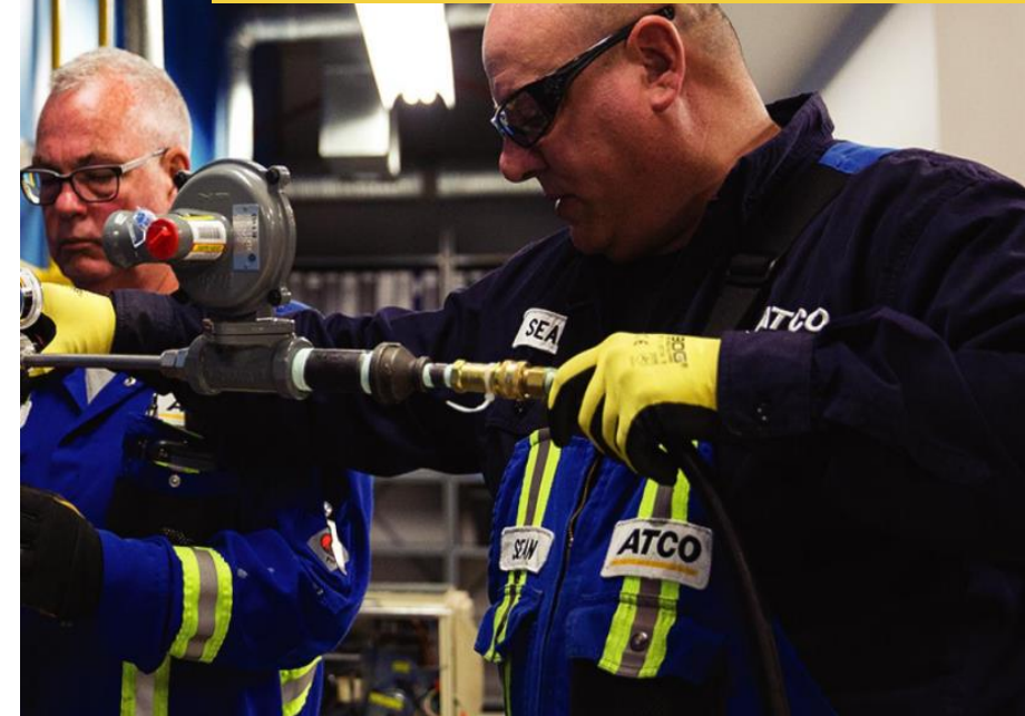
Hydrogen Blending Project - Alberta
