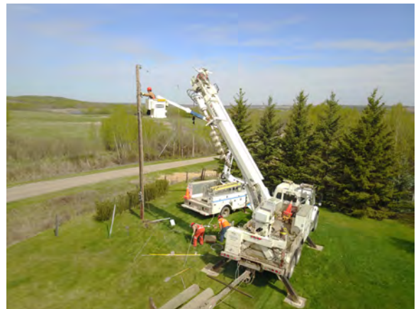
Electricity Distribution, Maintenance Work, Alberta
