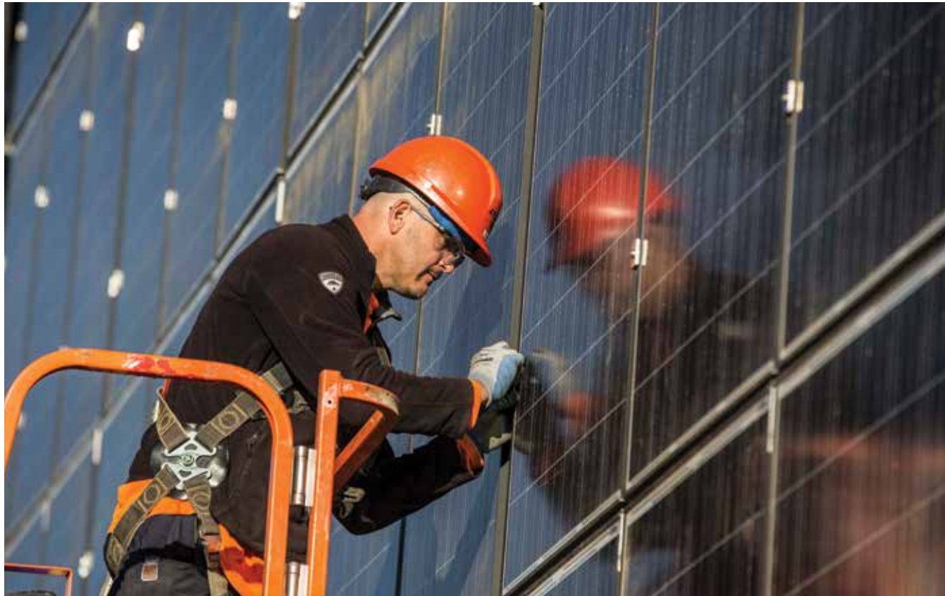
Our off-grid solar project at the Saddle Hills Telecommunications Site in northwestern Alberta is the largest in Western Canada, and is uniquely designed to provide reliable electricity in a remote northern environment.
