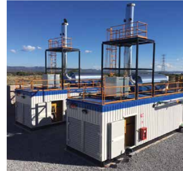
Our innovative distributed power generation solution will deliver up to 20 megawatts of reliable and efficient onsite electricity in a growing industrial park in Mexico.
