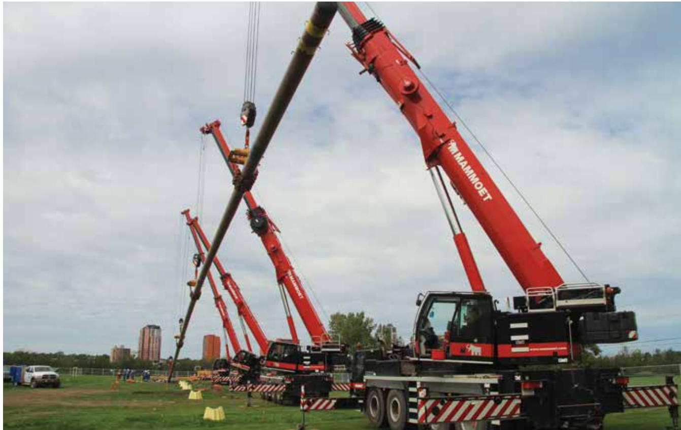
Our Steel Mains Replacement Program replaces aging steel pipe. In 2016, we replaced 41 kms of pipe through this program.
