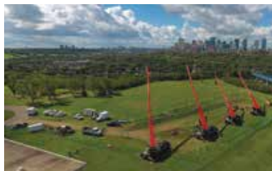
Crews prepare to replace steel mains on a natural gas pipeline servicing downtown Edmonton.
