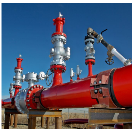
Natural Gas Pipeline Valve Assembly
