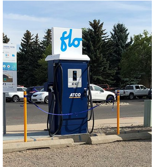
EV charging station, Lethbridge, Alberta
