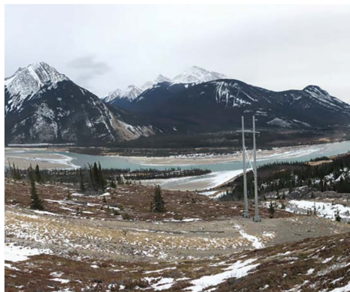
The Jasper Interconnection Project transmission line connects Jasper to Alberta's electric grid, providing safe and reliable power for residents and visitors.
