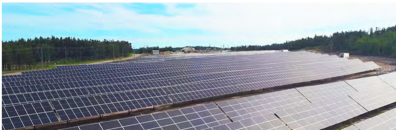
Fort Chipewyan Solar Project, Fort Chipewyan, Alberta
