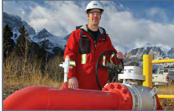
NATURAL GAS TRANSMISSION
