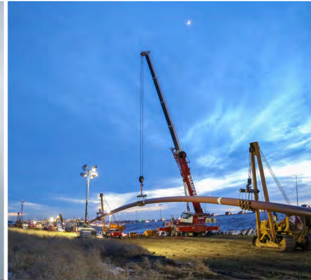
NATURAL GAS TRANSMISSION
