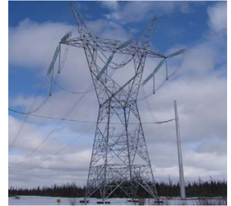
FORT MCMURRAY WEST 500 KV TRANSMISSION
