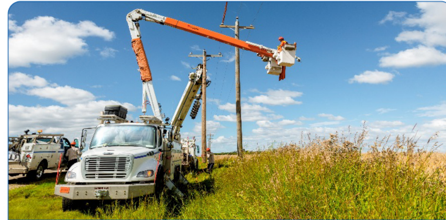
ELECTRIC DISTRIBUTION $2,585M Rate Base
