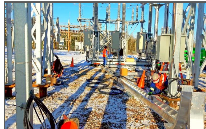
ELECTRIC TRANSMISSION $211M
